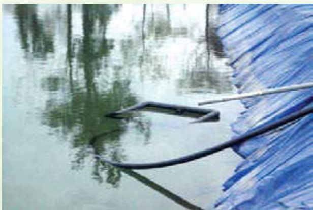
Fig. 10. Submersible Pump in Floating Platform
